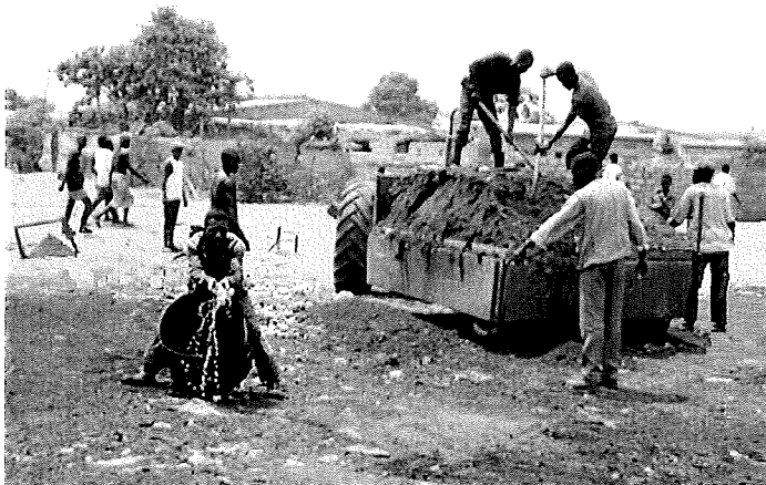
Figure 8 Road in-filling technique using water to increase the moisture content of the soil for better compaction.
